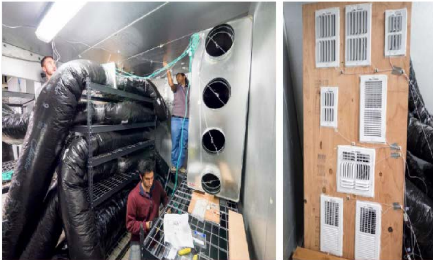
Fig. 3. Layout of ducts and grilles in the outdoor environmental chamber at the Western Cooling Efficiency Center, University of California – Davis.
