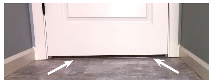
• Install a return air pathway or 1" door undercut at bedrooms with only one supply and no dedicated return.
