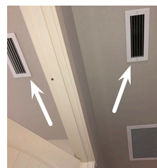
• Final Jumper Duct
