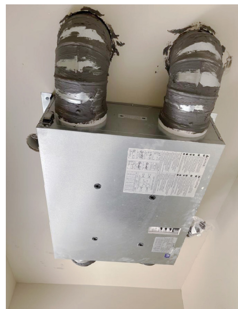
• Heat Recovery Ventilator (HRV) or Energy Recovery Ventilator (ERV)
