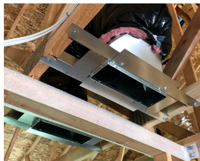
• Rough Jumper Duct
