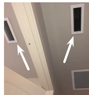
• Final Jumper Duct
